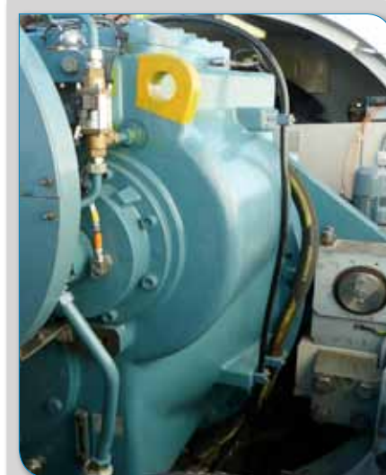
AC accelerometers can be used to identify gear defects.
